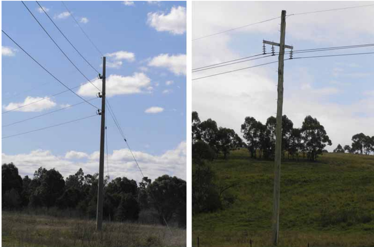
Figure 5 Photographs of single pole structures on 66kV power lines.
