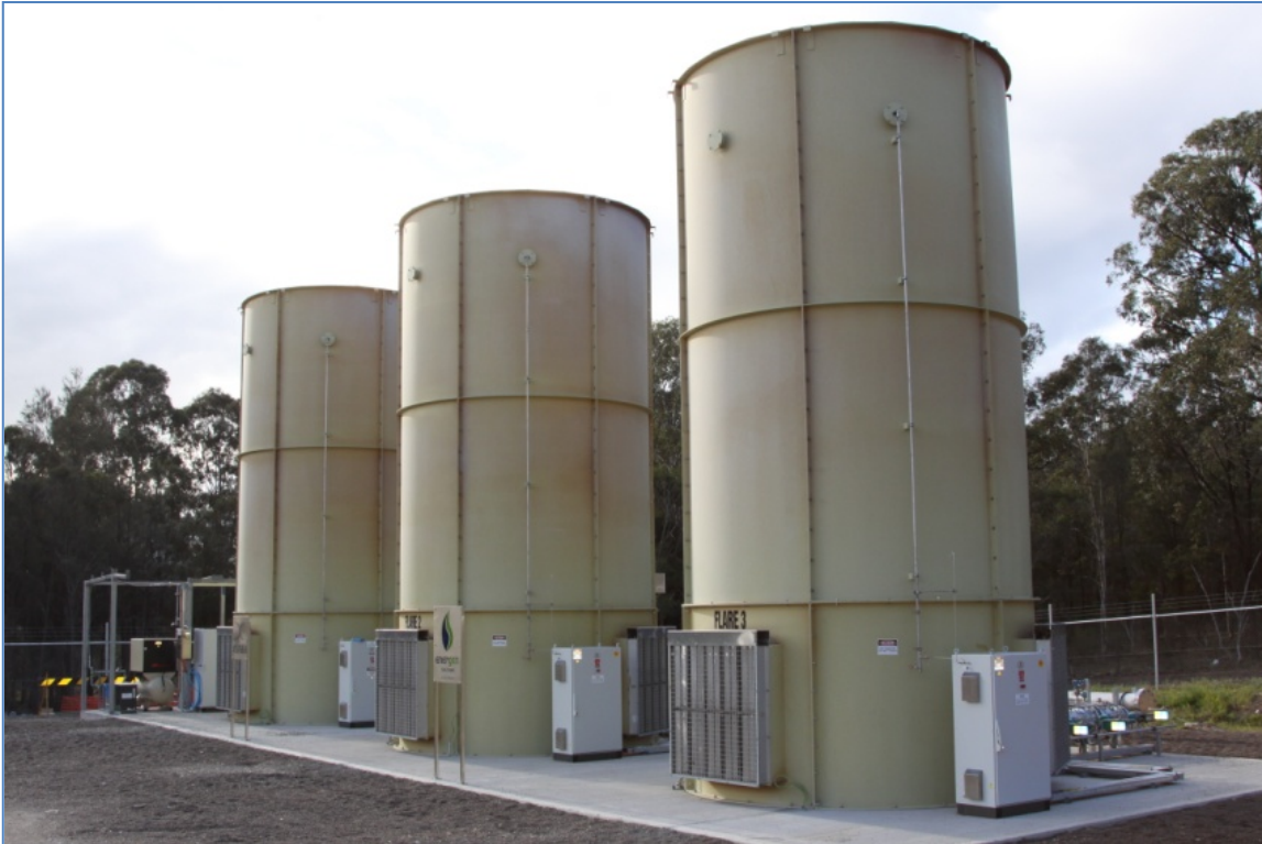
Photograph 4: Enclosed flares in use at another underground mine
