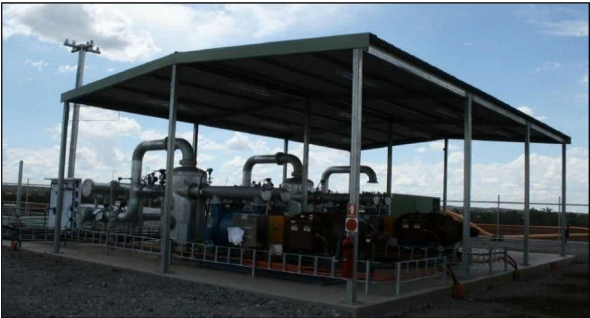
Photograph 3: Example gas drainage plant (as used at another NSW coal mine)
