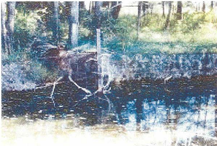
Figure 3. An intact section of engineered channel in Bowmans Creek showing the railway line piles, cables and mesh holding a constructed gravel bank.
