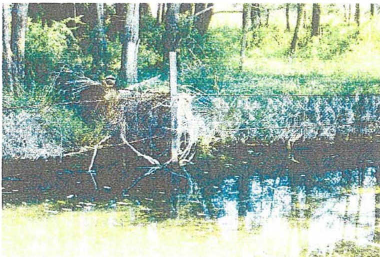
Figure 3. An intact section of engineered channel in Bowmans Creek showing the railway line piles, cables and mesh holding a constructed gravel bank. GR 317858E 6406286N
