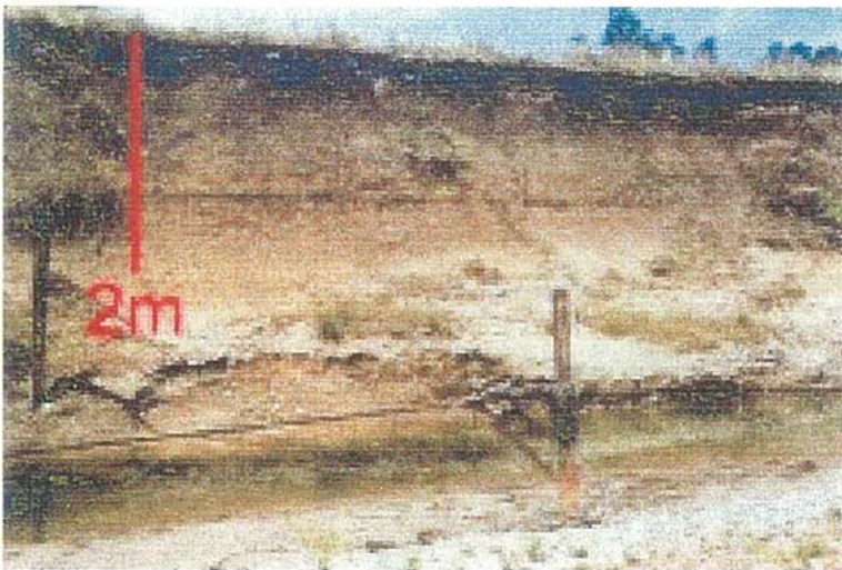
Figure 5. A section of engineering works that has failed where the face of second terrace is being eroded. Bowmans Creek upstream of the highway bridge. The surface of the terrace has nearly 60cm of PE sediment over silty clay alluvium.
