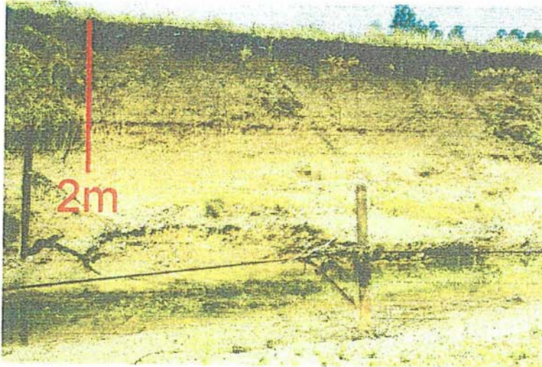
Figure 5. A section of engineering works that has failed where the face of the second terrace is being eroded. Bowmans Creek upstream of the highway bridge. The surface of the terrace has nearly 60cm of PE sediment over silty clay alluvium. GR 6406883N 318433E
