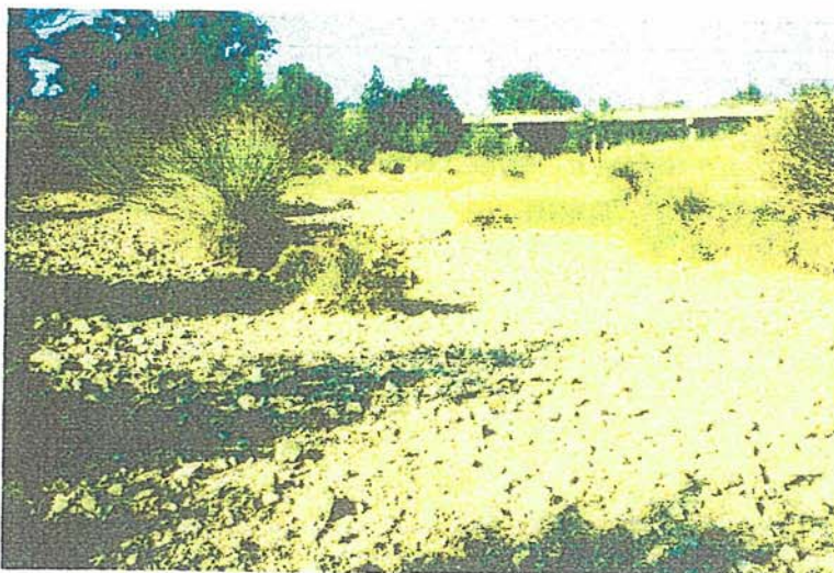
Figure 6. Bed and part of the low floodplain of Bowmans Creek upstream of the highway bridge showing the effects of recent scour. Even small floods are moving pebbles up to 25cm in diameter as bed load. GR 318455E 6406473N
