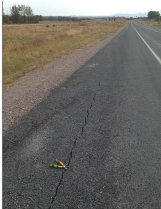
Figure 6 Lemington Road cracking FROM LW6B panel
