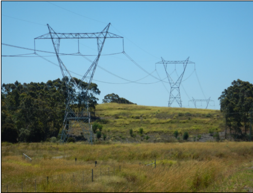
Plate 1: TransGrid 330 kV Transmission Line along western boundary of Extraction Plan Area
