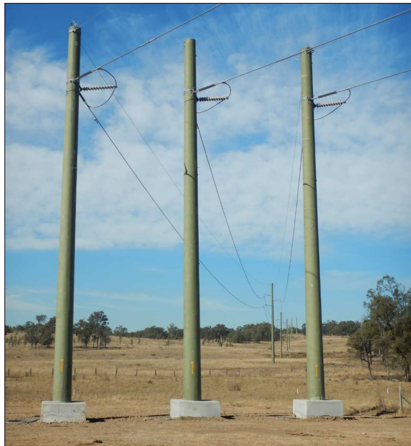
Figure 3: Set 9 at change of direction with concrete pad footings in position (Set 29 in background).
