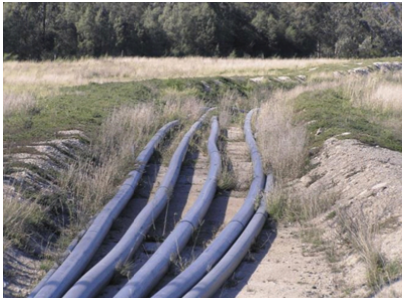
Plate 1: ACOL Tailings Disposal Pipelines in Open Trench
