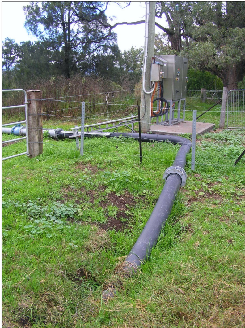
Figure 17: ACOL water supply pipeline.
