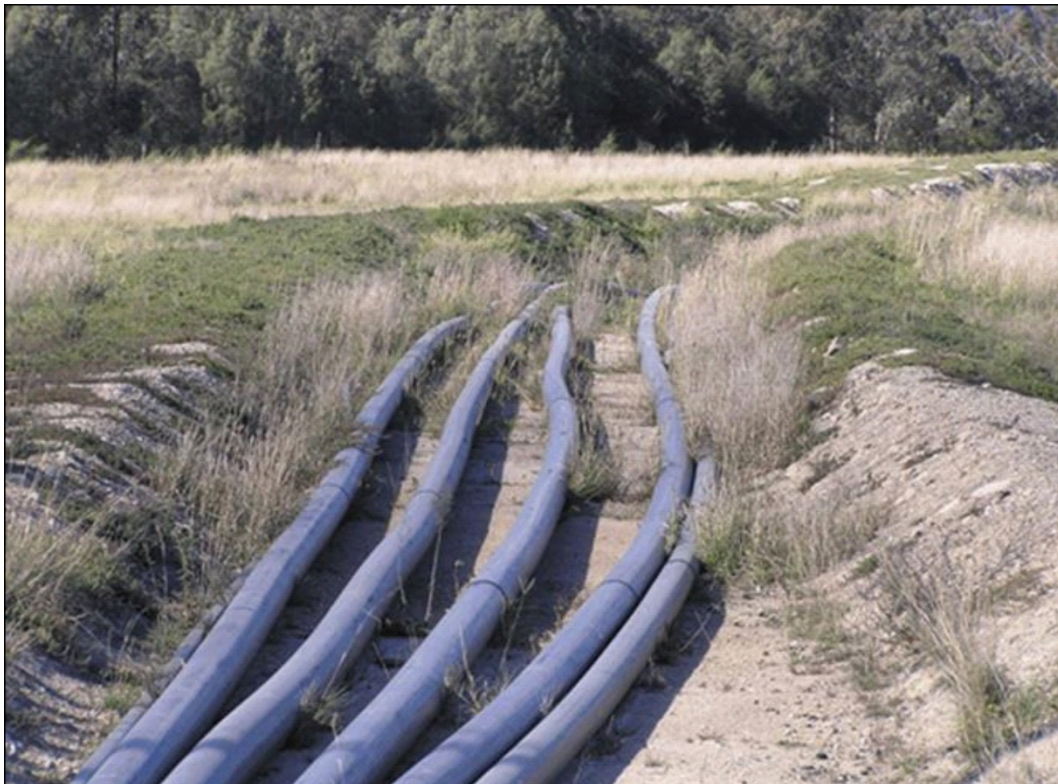
Figure 16: ACOL tailings disposal pipelines in open trench.
