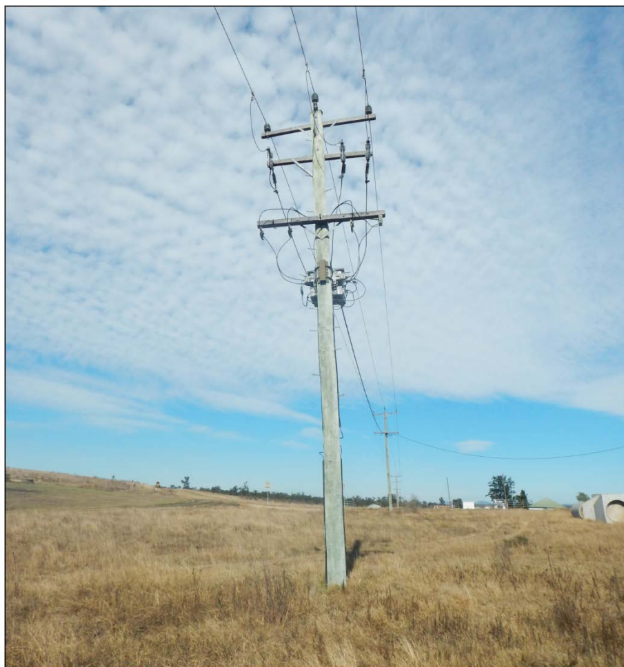
Figure 13: 11 kV powerline over the northern section of Longwall 204.
