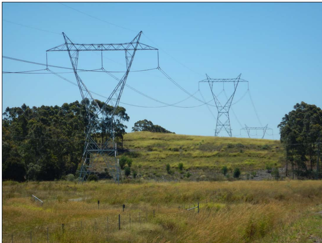
Figure 14: 330kV Transgrid Power Transmission Line.
