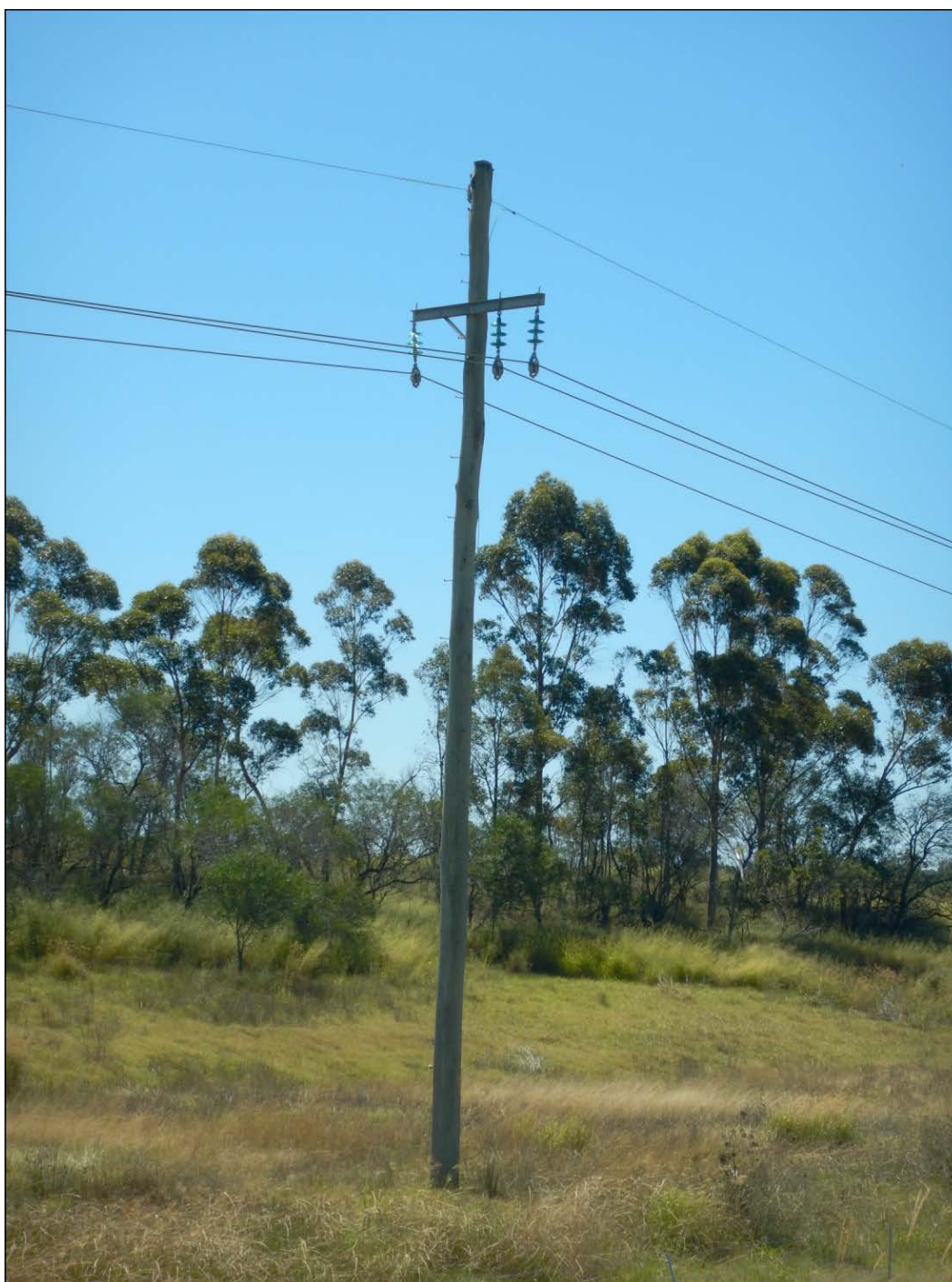
Figure 17: 33kV Local Power Transmission Line.
