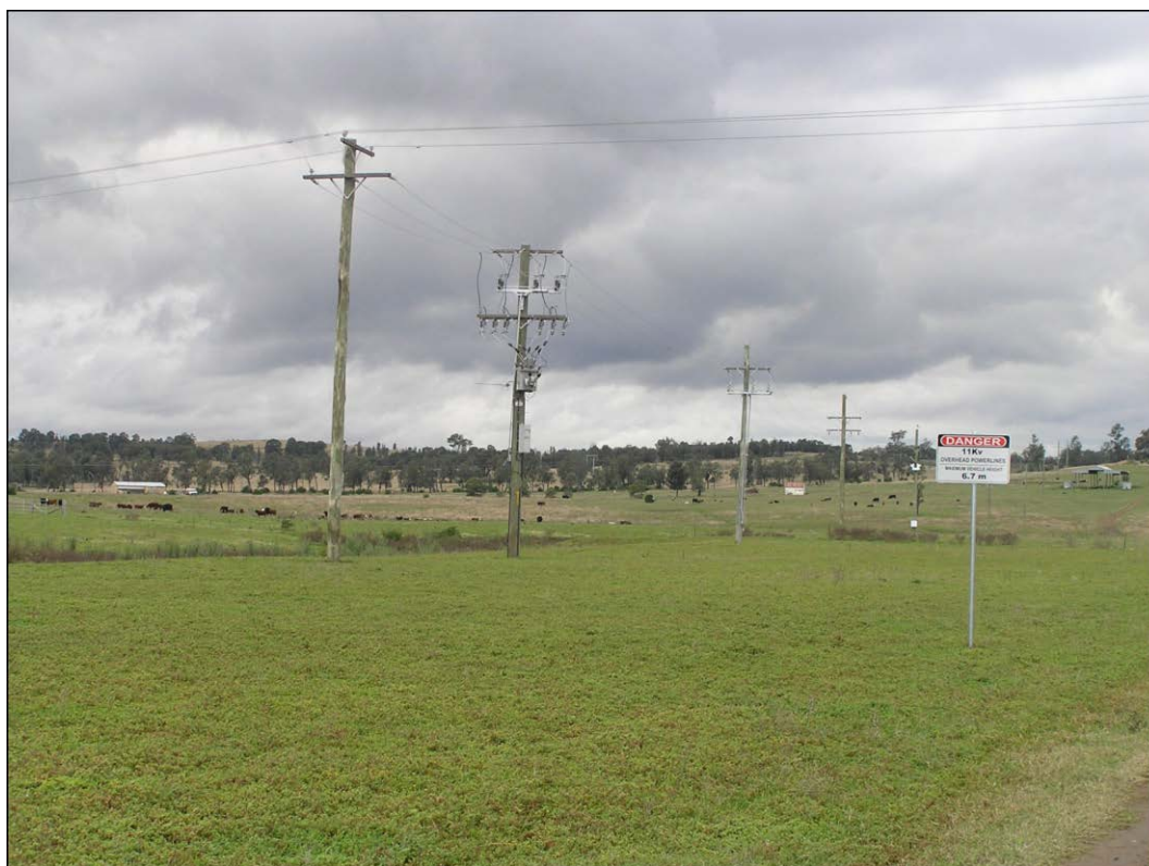
Figure 16: 11kV Local Power Transmission Line.
