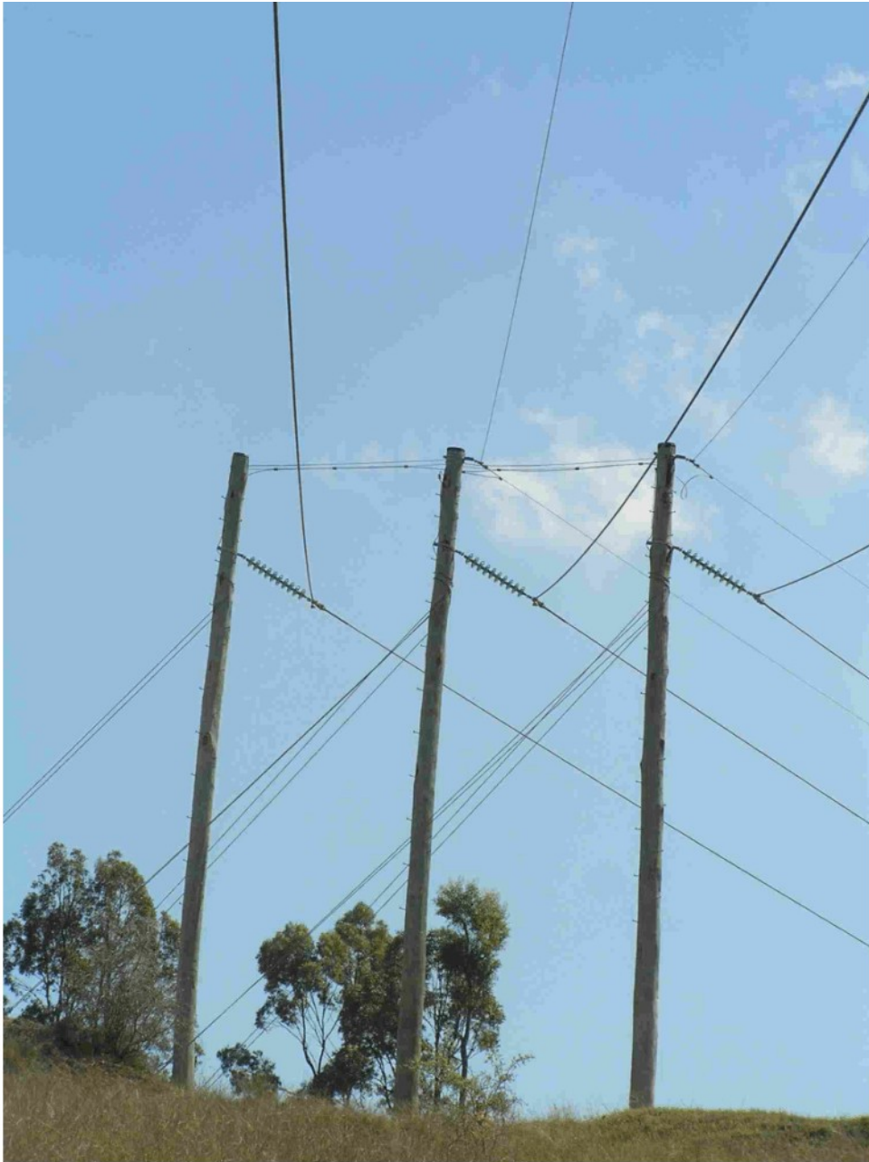
Figure 16 Three pole structure at the change of direction of 132kV power line over Longwall 2.
