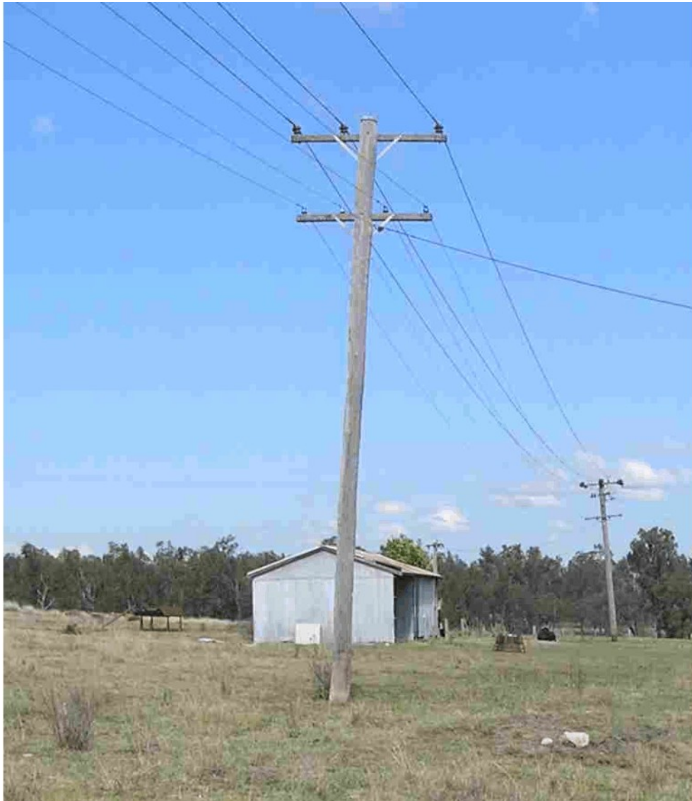
Figure 13 Local distribution power line supported on single pole structures at the northern end of Longwall 4.
