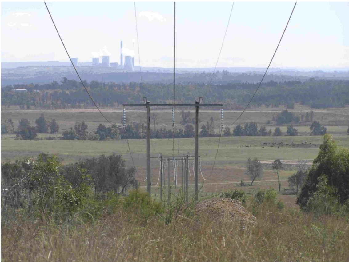
Figure 15 132kV power line traversing the southern end of the SMP Area looking west.
