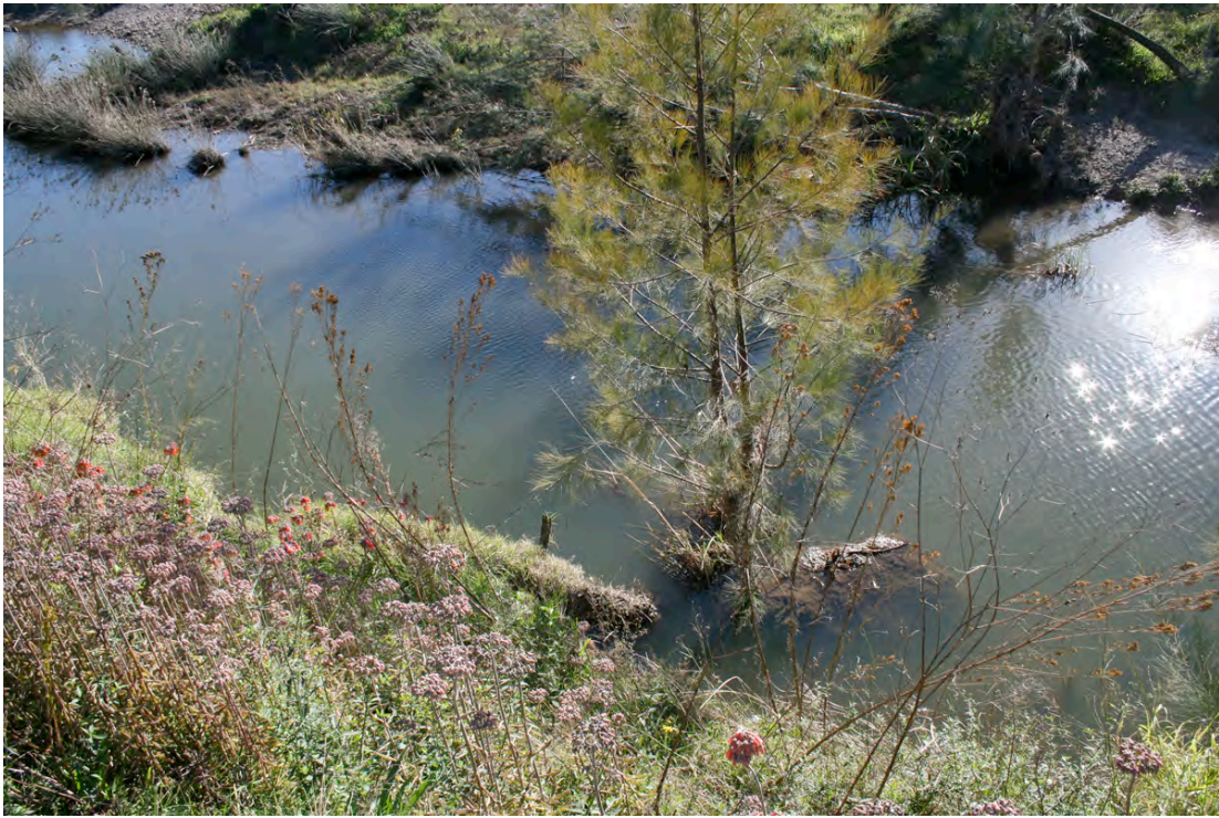
Photo 3: Looking down from top of eastern bank at eroded bank section (July 2008).
