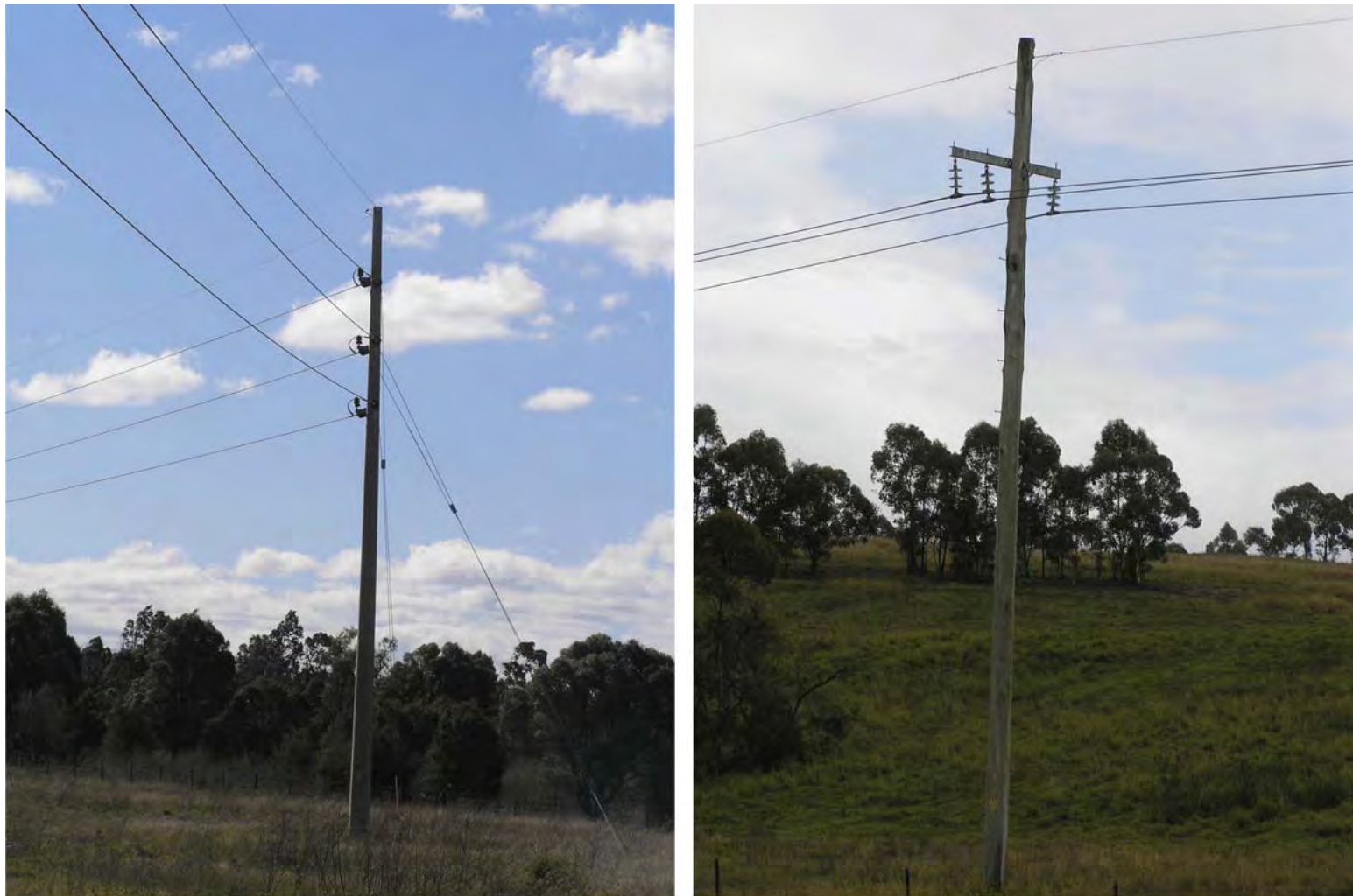
Figure 10 Photographs of single pole structures on 66kV power lines.
