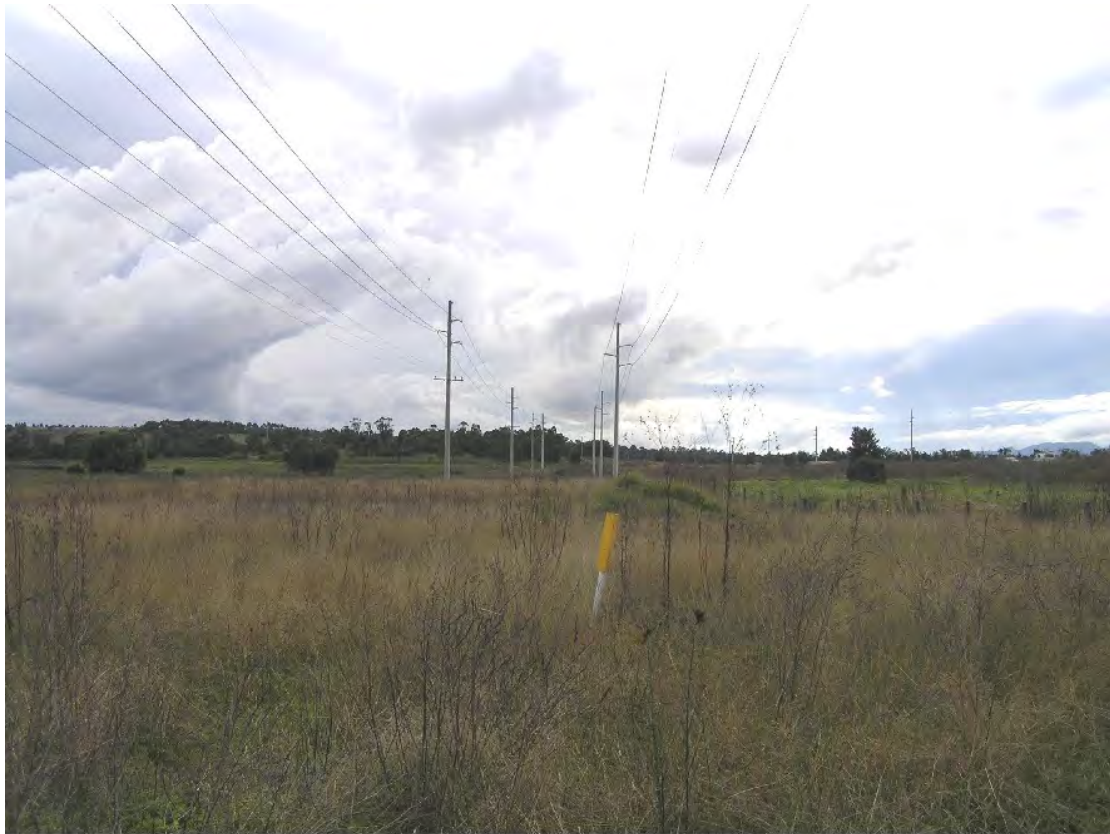
Figure 8 Photograph of Powertel cable and high voltage power lines in New England Highway road reserve.
