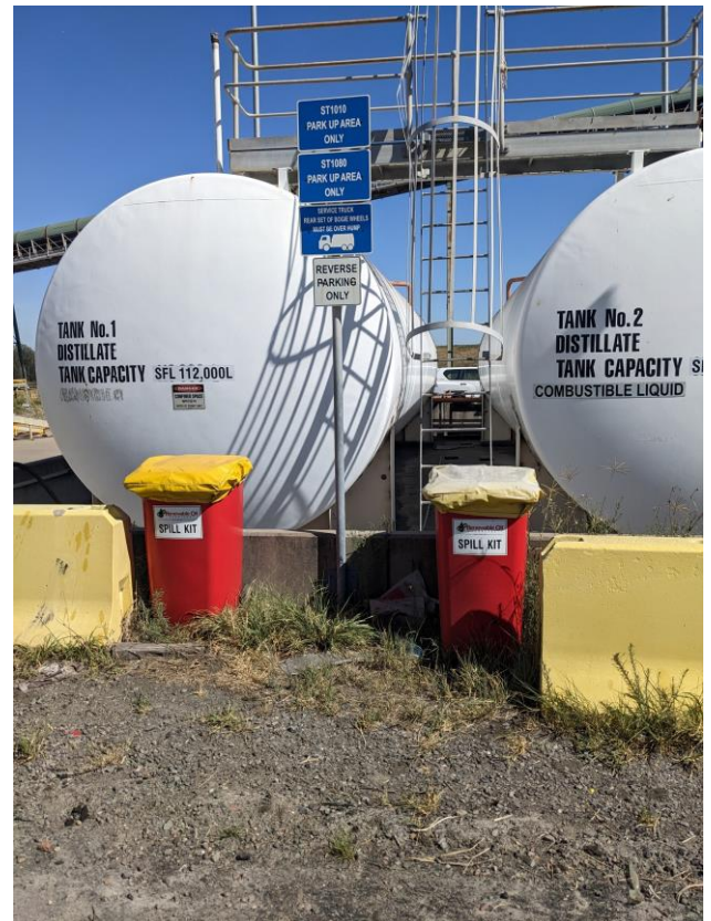
Plate 4.2 Bunding and spill kits around dangerous goods storage
