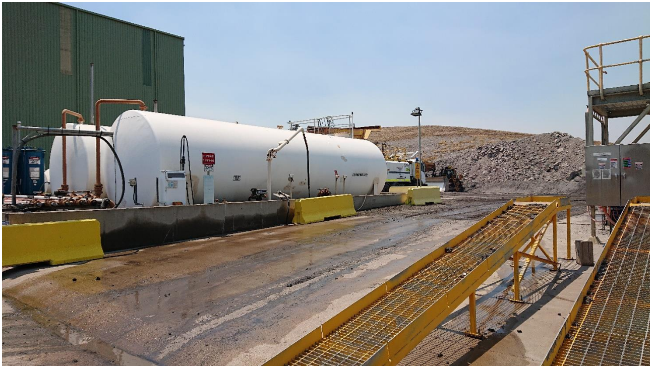
Photo # 3 - Fuel Storage (Heavy Plant Maintenance Area)
