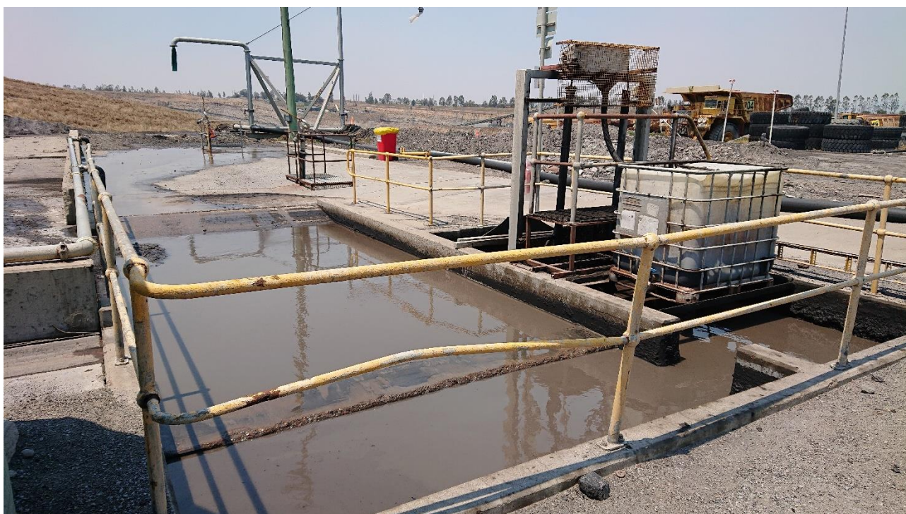
Photo # 11 - Plant wash down with oil water separator
