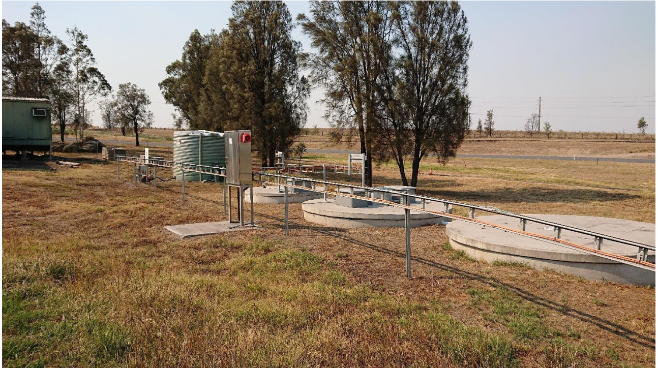
Photo # 8 - Sewage Treatment Plant
