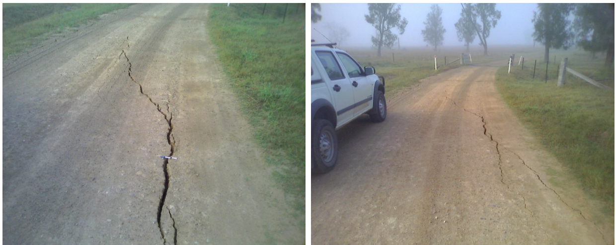
Figure 14. Subsidence cracks, Longwall 3
