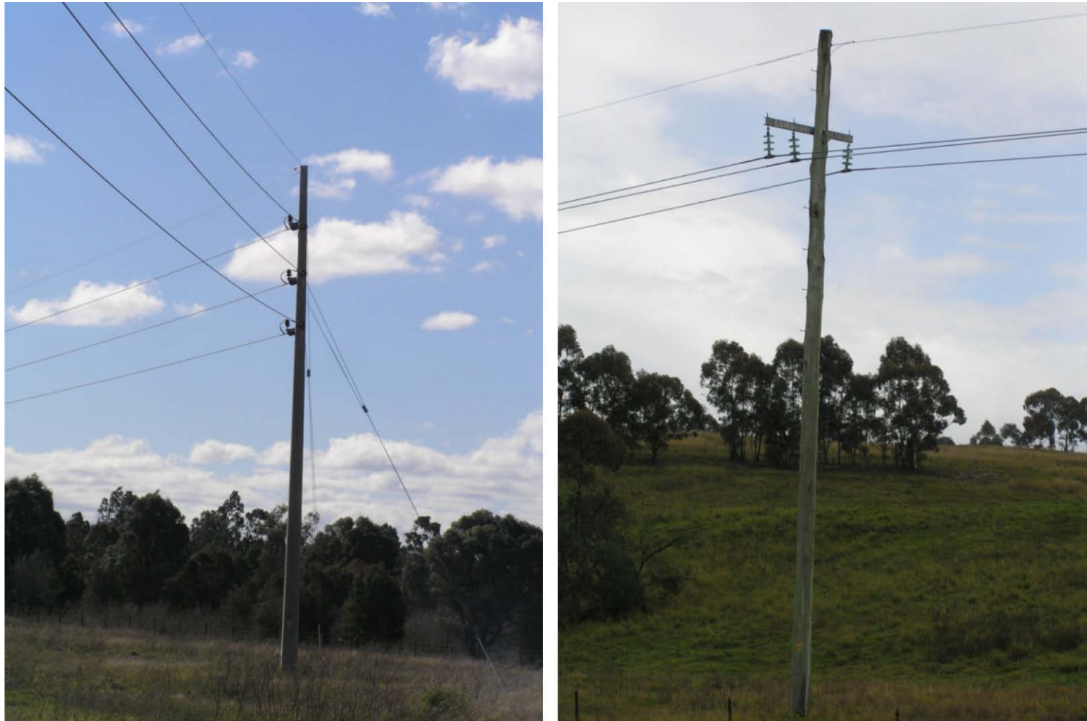
Figure 12: Photographs of single pole structures on 66kV power lines.
